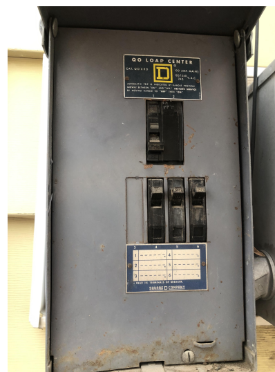
Figure 6: Electrical panel detailing 100A service specification. Also, throughout the house tour, measurements were taken for the windows to make an estimate on equipment requirements and available rebates. The ASHP installer we spoke to recommended a mini-split
